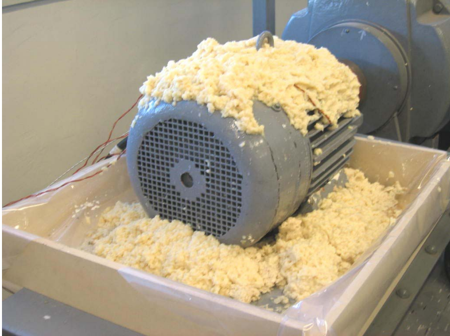
Fig. 5. Motor without cover and pulp spilled over it; clean air intake area
